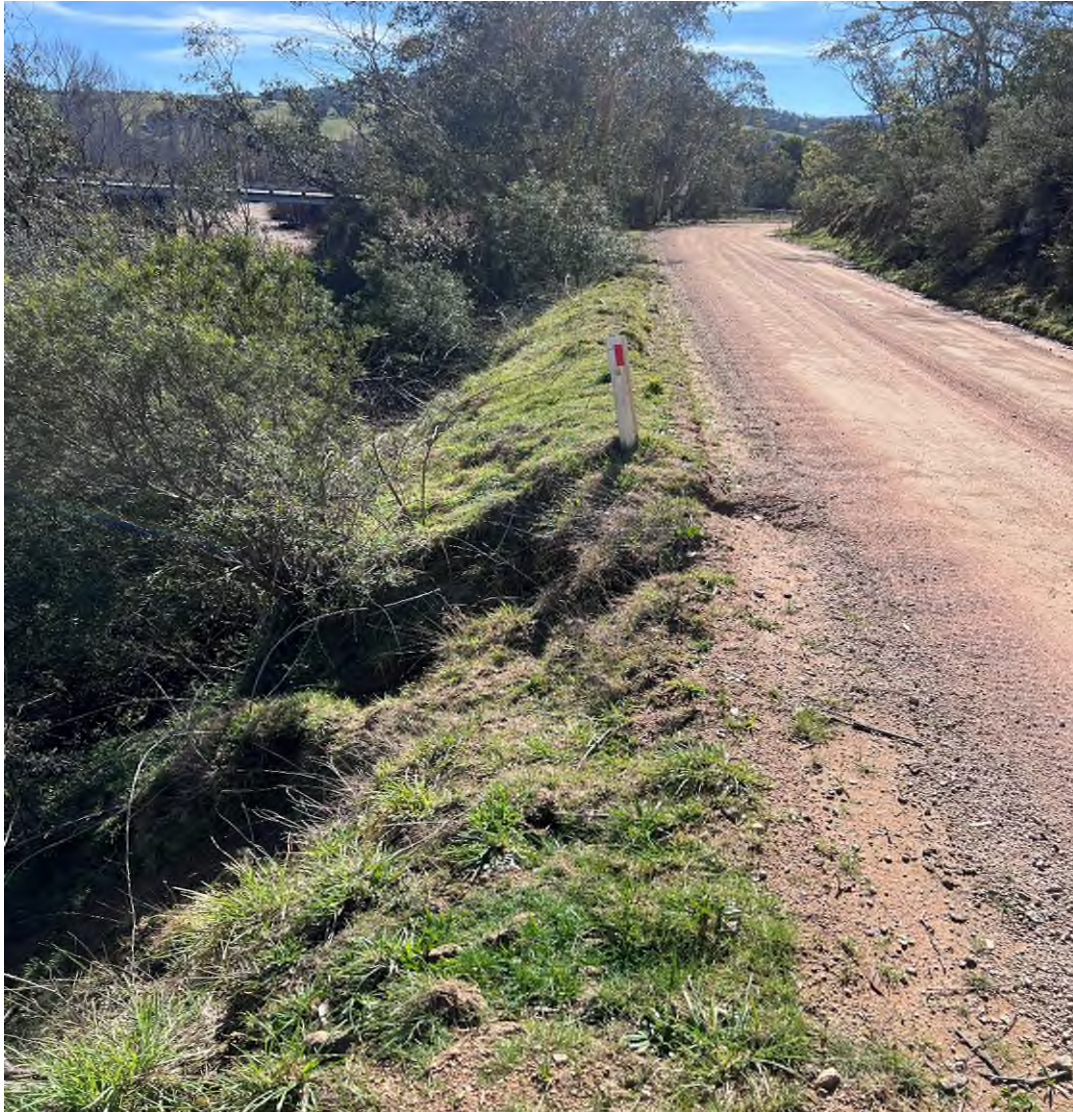
Figure 4: Wallace's Gap Road – Erosion Risk Areas Where Slope Stability Analysis Required
